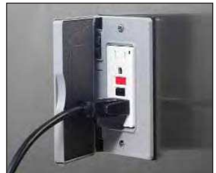
Electrical duplex receptacle with splash cover
